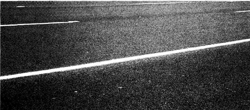
PHOTOGRAPH 6. APPEARANCE OF STONE MASTIC ASPHALT (SMA 3) TEST SECTION AFTER ONE WEEK. (Note the coarse (open) surface texture of the SMA 3 shoulder and driving lanes in the foreground compared to the conventional dense friction course (DFC) passing lane in the background.)
