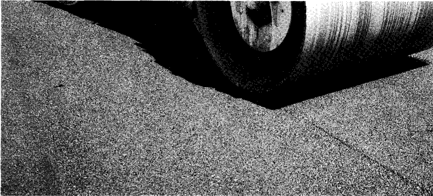
PHOTOGRAPH 5. COMPACTION OF STONE MASTIC ASPHALT (SMA 3) TEST SECTION. (There were no problems in producing (with extended dry mixing time), placing and compacting the SMA 3 mix. Static steel-wheel compaction is used to avoid potential fracture of coarse aggregate with vibratory compaction and surface flushing of mastic with pneumatic compaction. A soap solution should be used with rollers on SMA mixes containing polymer modified asphalt cement.)
