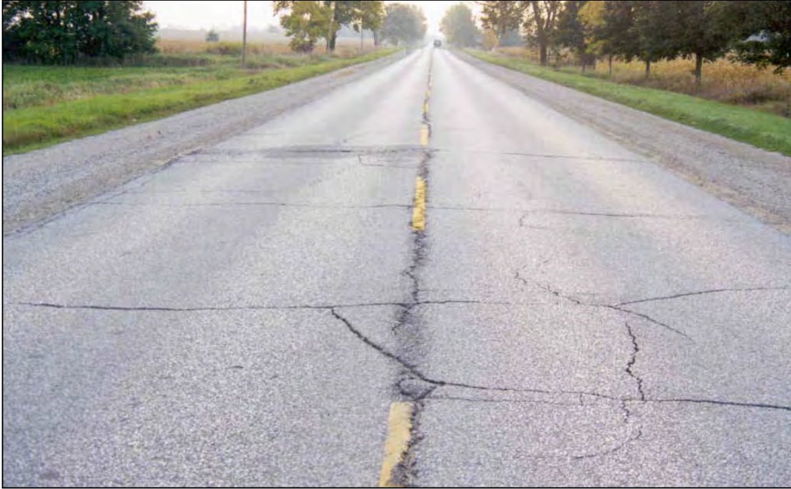
Photograph 1: Typical condition of County Road 2 prior to rehabilitation
