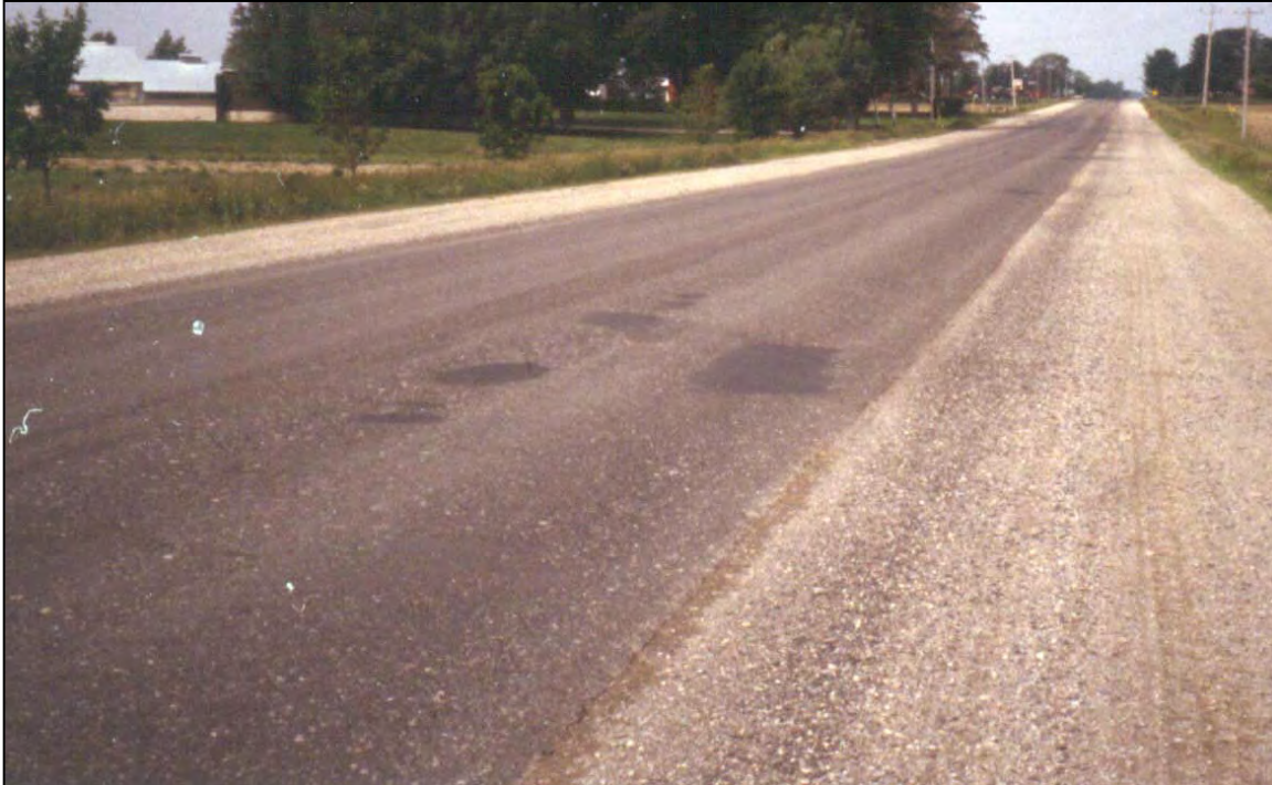
Photograph 2: Raveling of recycled mat leading to potholing
