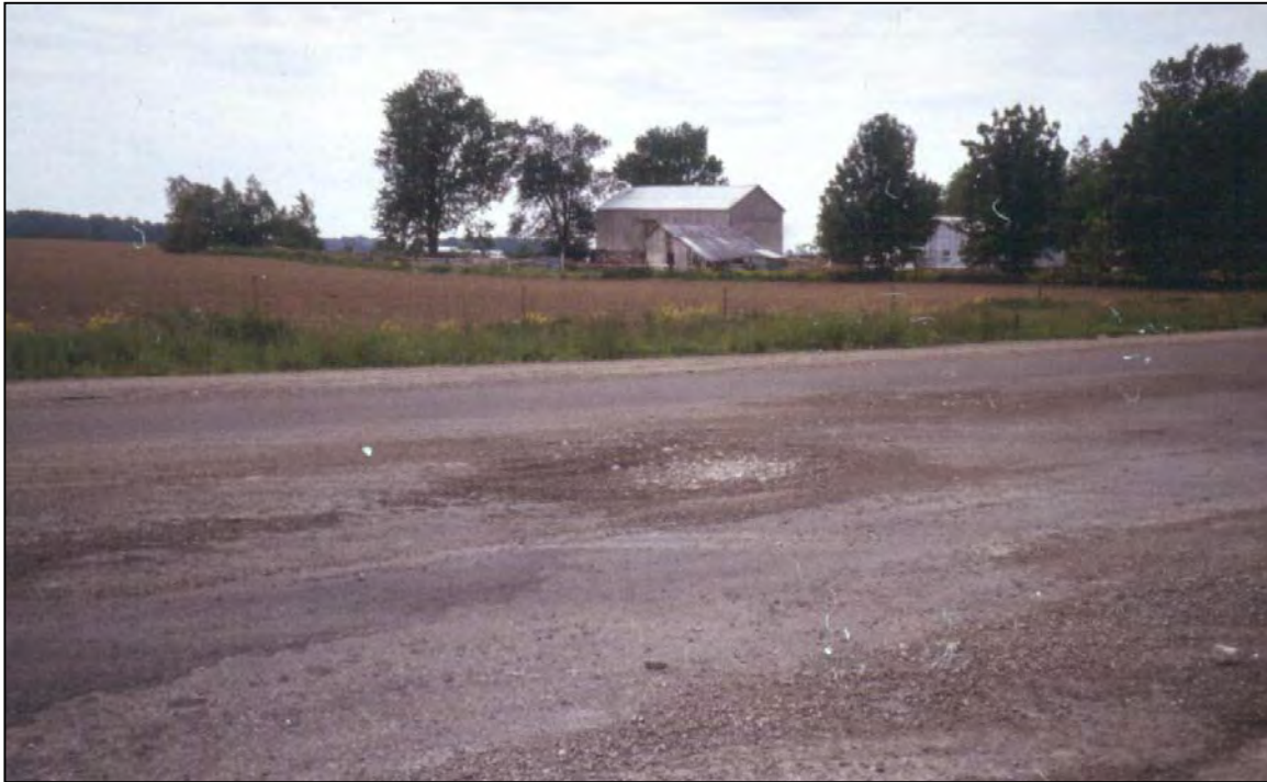
Photograph 3: Localized rapid breakup of recycled mat
