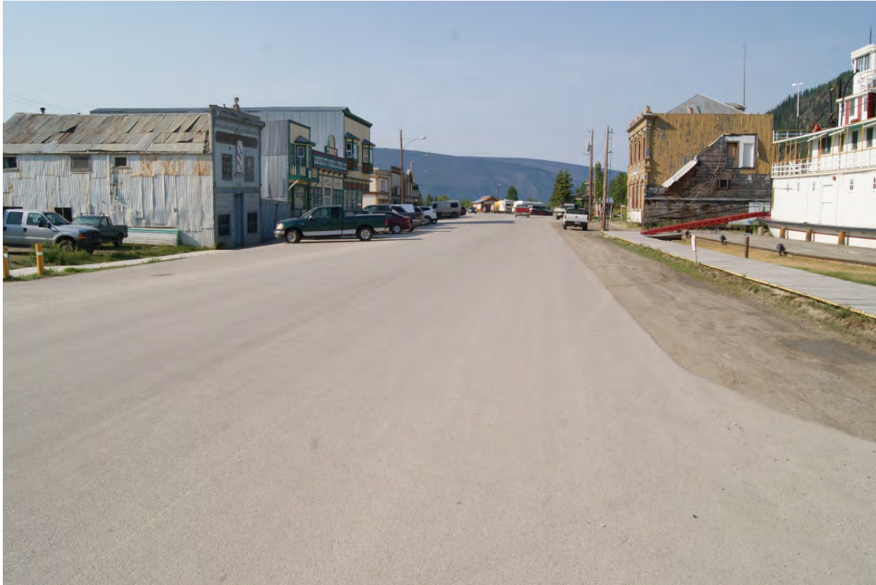
Figure 5. Front Street Pavement Conditions as of May 2015
