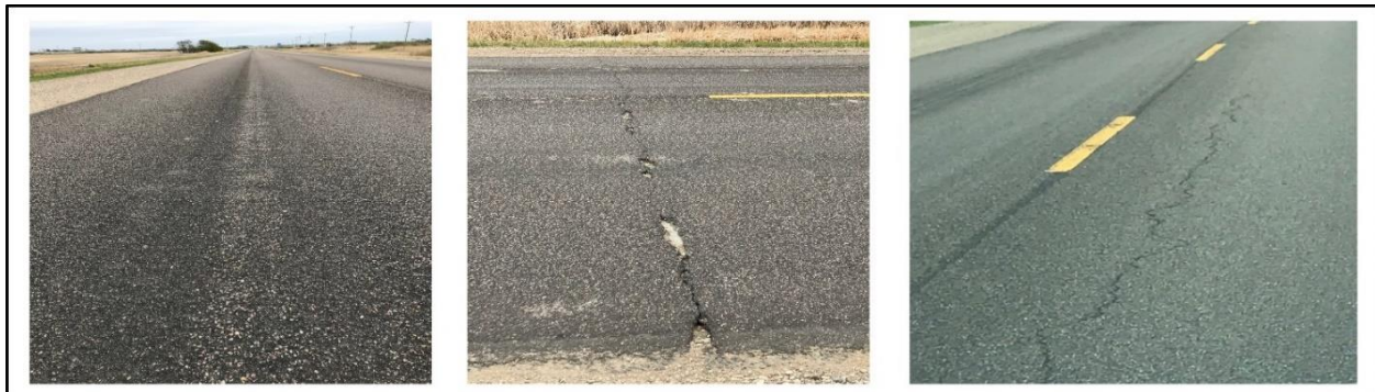
Figure 8. Highway Section Completed Using Job Mix E III in South Western Manitoba
